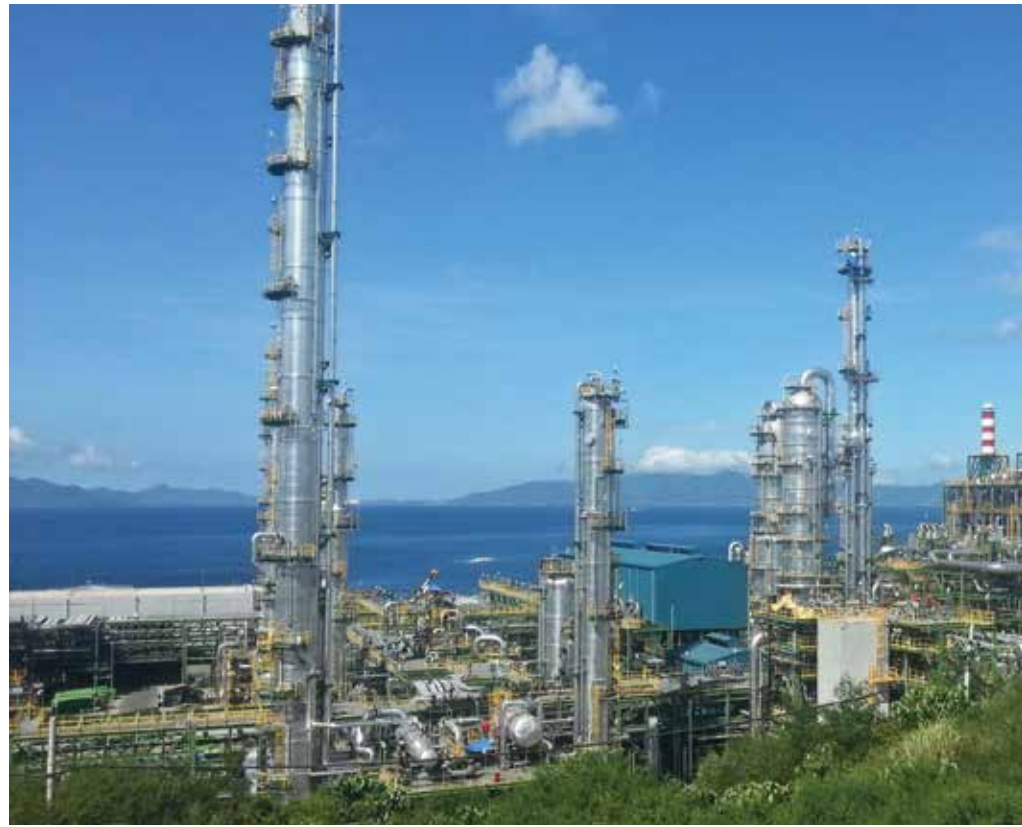
This Naphtha Cracker plant located in the Philippines is the home of several of the largest Velan air-operated gate and globe valves ranging from 1" to 24". These valves are designed for either fail-open or fail-close operation which are very critical parts of the process.
