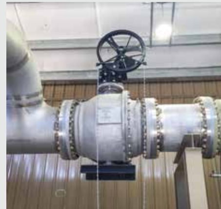
30" 150# API 6D SSTMV Installed in CO2 Recovery Unit.
